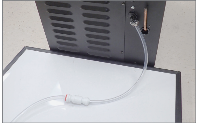
FIG. 5. Installed check valve.
